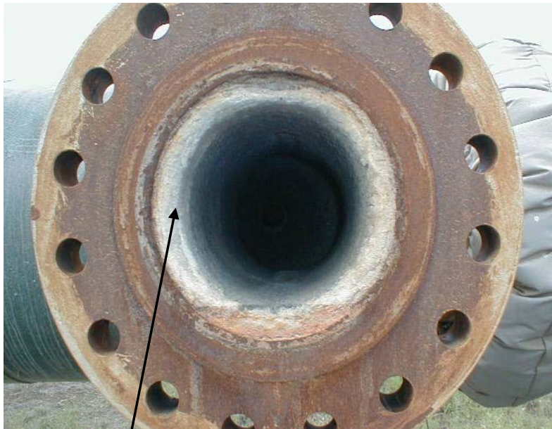
Thickness of scale deposited in two-phase line. 1 inch thick
